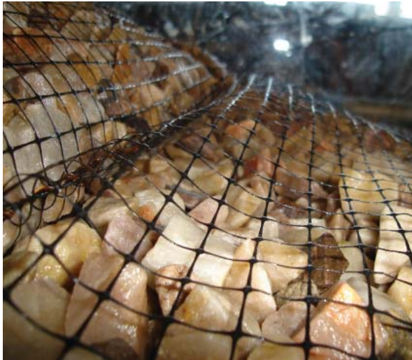
Figure 5.15: Bulging of a compartment
