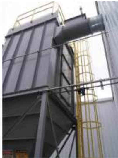
Figure 11a: Dust collector before the deflagration (Luzik, 2015)
