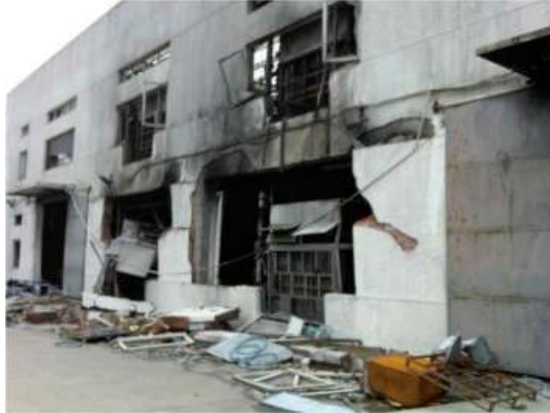
Figure 7d: Damage to the eastern wall of the main building (Li et al., 2016)
