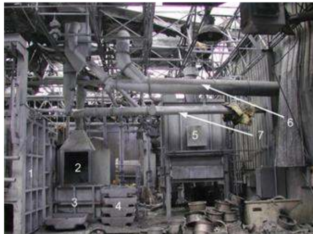
Figure 6c. Damage to the interior of the facility (Chemical Safety Board, 2005)
