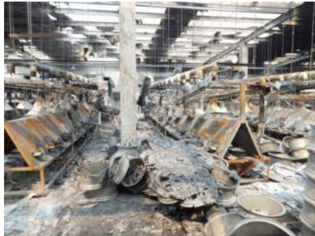
Figure 7c: Damage to the production lines and work stations (Li et al., 2016)
