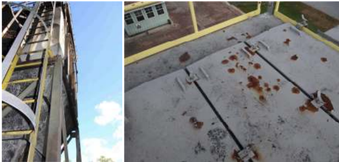
Figure 11d and 11e: Dust collector after the deflagration: deformation of the reinforced wall and access doors (Luzik, 2015)
