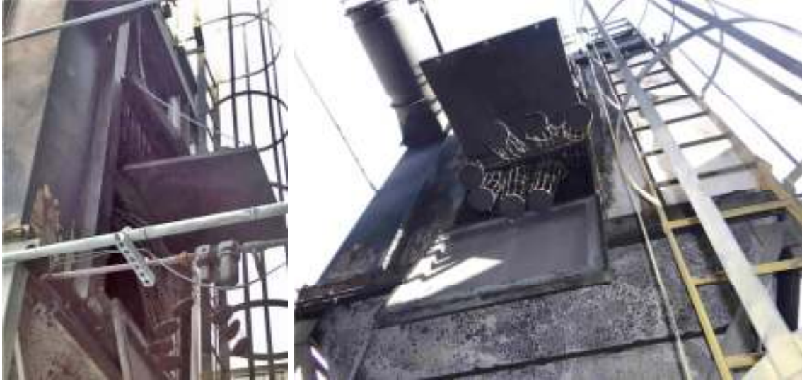
Figures 11b and 11c: Dust collector after the deflagration: filters blown through the vents (Luzik, 2015)
