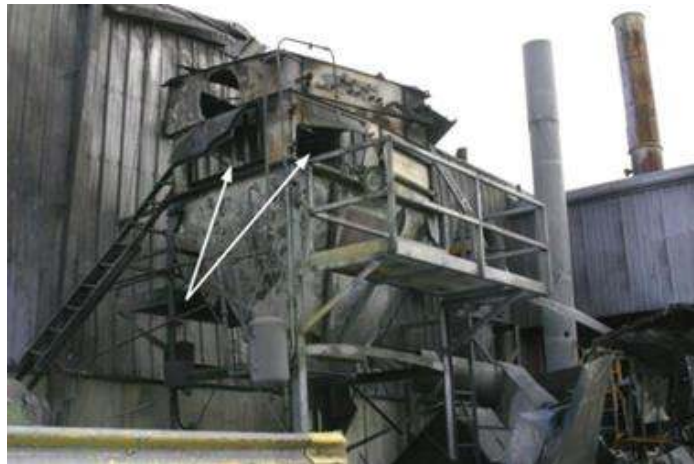
Figure 6a. Damage to the dust collector (Chemical Safety Board, 2005)
