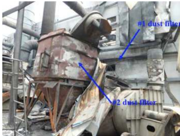
Figure 7b: Damage to the dust collectors (Li et al., 2016)
