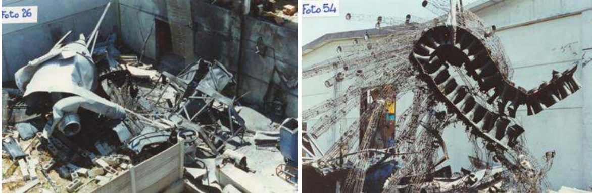
Figures 4b and 4c. Bagfilter before after the aluminum dust explosion (Marmo et al., 2015)
