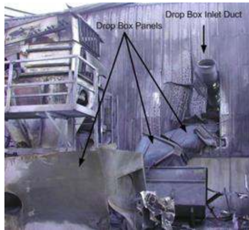
Figure 6b. Damage to the drop box (Chemical Safety Board, 2005)
