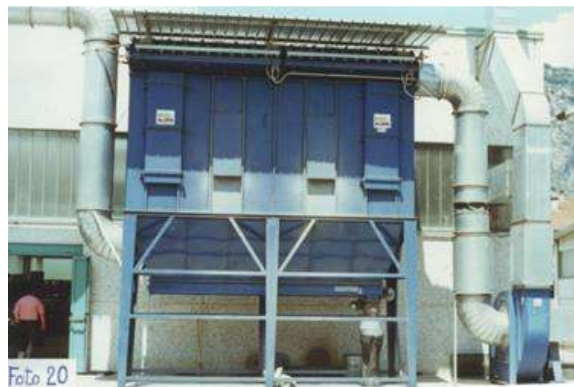
Figure 4a. Bagfilter before the aluminum dust explosion (Marmo et al., 2015)
