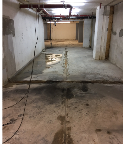
Figure 32: Unexpected situation in the structure of the basement. A junction which was constructed may cause stability issues in the future
