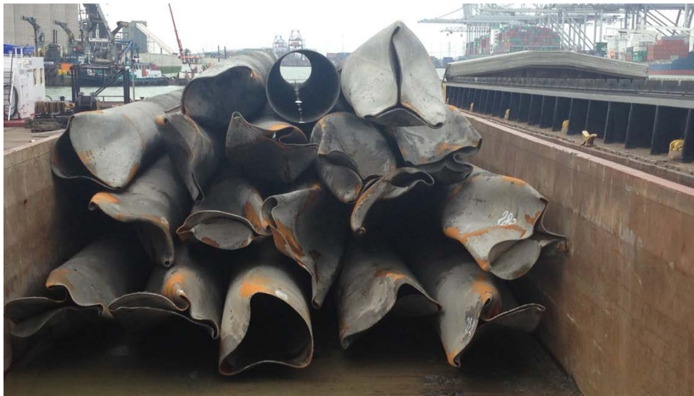
Figure 9: Heavily damaged pile toes
