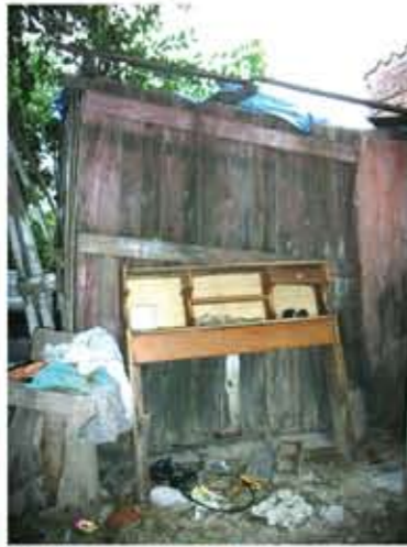
On the left the old kitchen which is located behind the first construction. This kitchen is no longer in use, because of the large number of holes in the roof.
