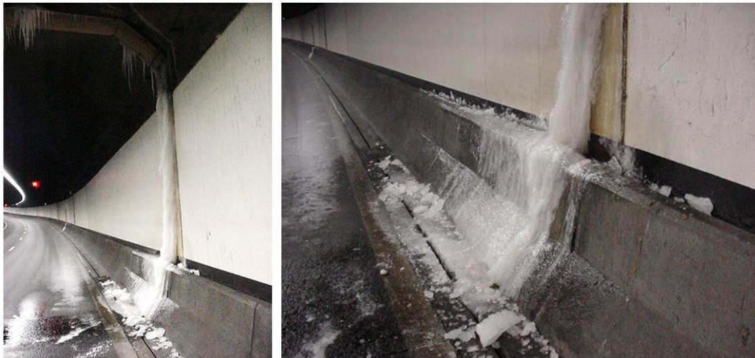
Figure 1: A leakage in the Drechtunnel in 2002 resulted in ice on the road and icicles on the roof, when the temperature was below zero degrees Celsius (Leeuw, 2008).
