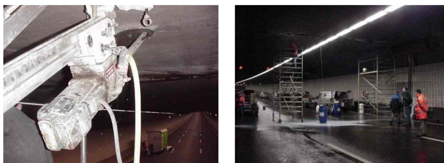
Figure 51: Injecting a leakage in the roof of a segment joint in the Noordtunnel (Leeuw, 2008).
