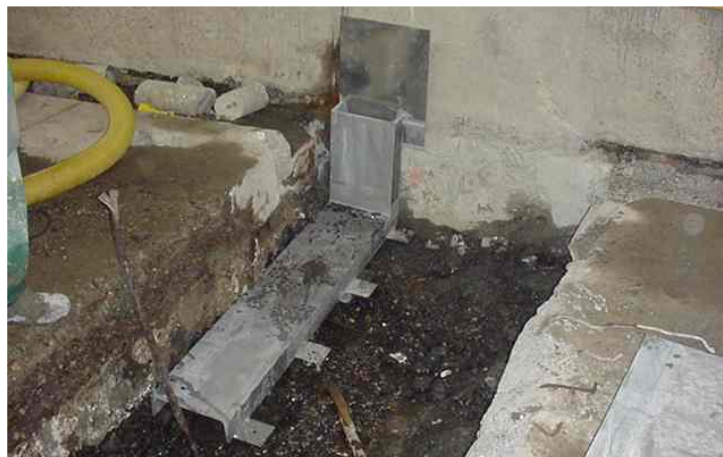
Figure 54: Drainage channel in the segment joint of the 1 st Heinenoordtunnel to solve the leakage of 4-5 m 3 /h (Leeuw, 2008).
