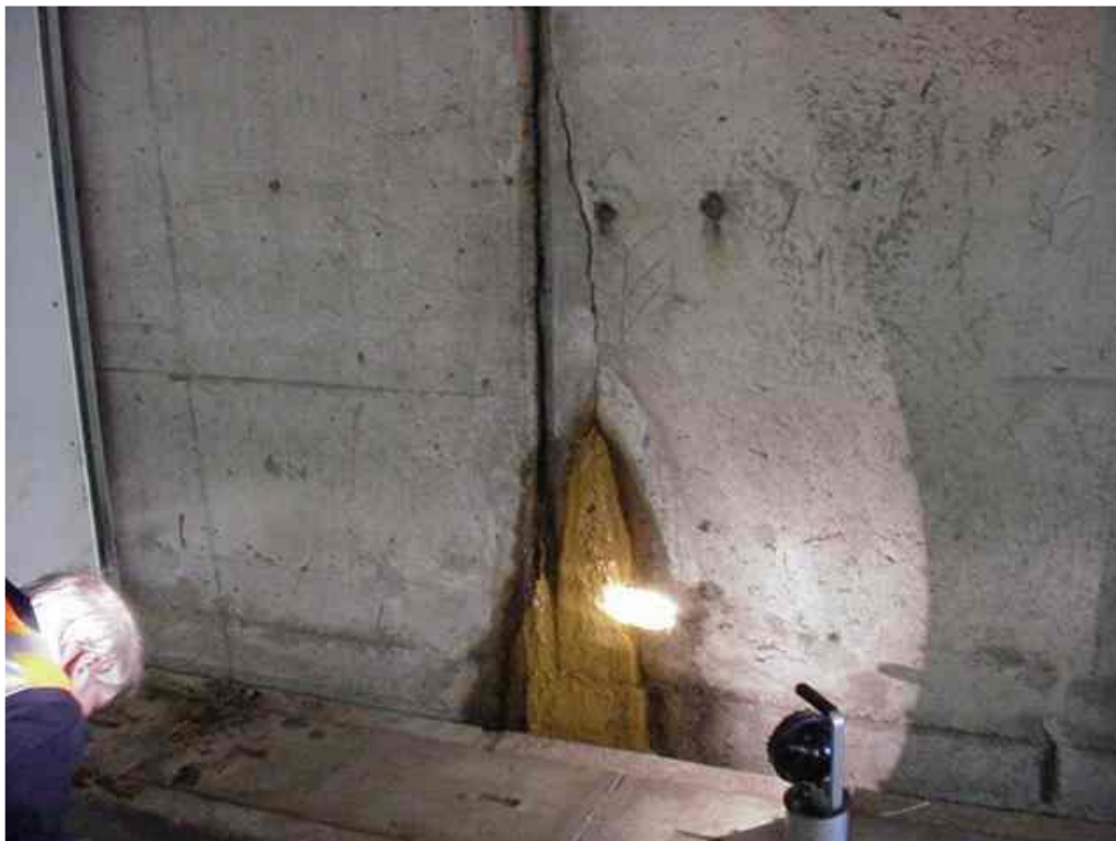
Figure 4: Leakage in the outer wall of a segment joint in the Kiltunnel, where foundation sand was transported into the tunnel (Leeuw, 2008).
