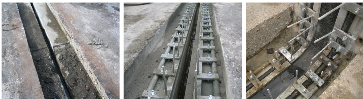
Figure 53: A new waterproof gasket is installed for the Roosendaal underpass A58 (Leeuw, 2008).
