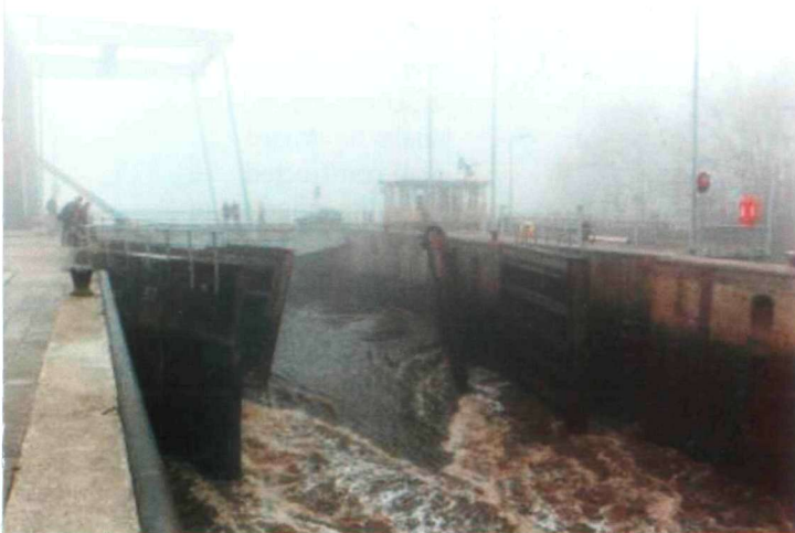
Figure 4 Failing structure at Delfzijl due to human error
