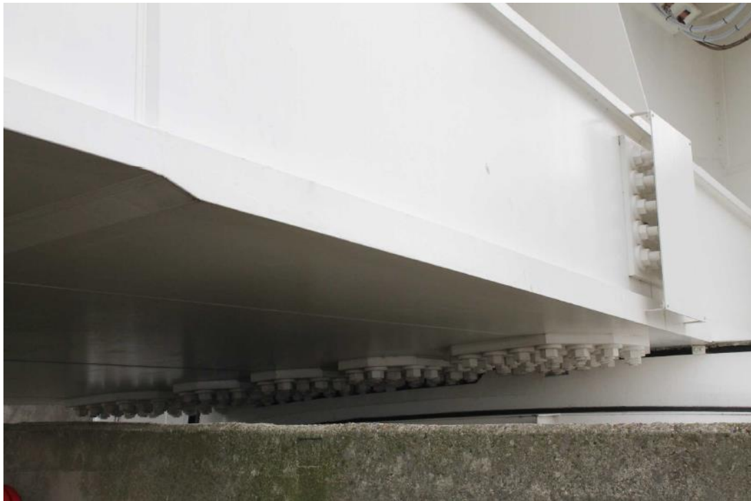
Figure 2.12: Image of connection between trusses and ball bearings with injection bolts in Maeslant Storm Surge Barrier [5]
