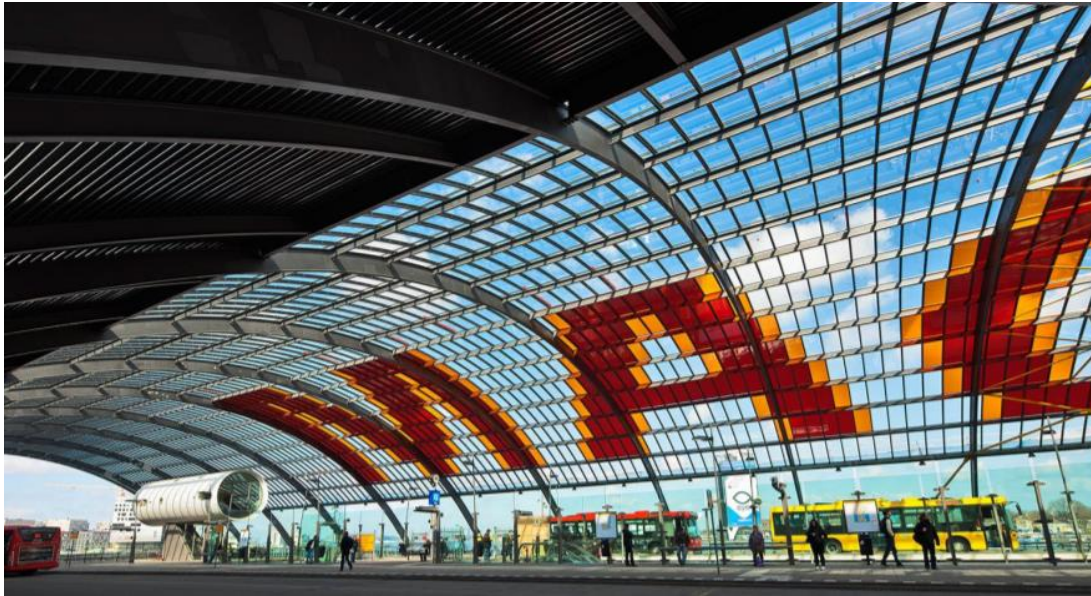
Figure 2.15: View of the glass roof steel structure from the inside of bus station [24]
