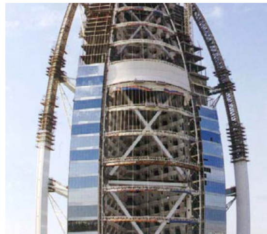
2.03 View on the atrium during construction time; giving a sense of the size of the atrium and its textile façade
