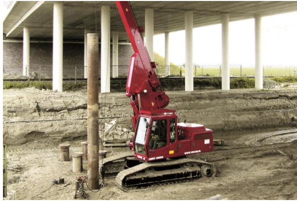
Figure D-3 Impression of a steel pile being installed by a free-fall drop hammer inside the pile (Vroom, 2016)
