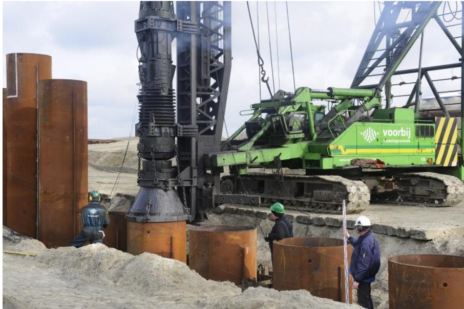
Figure D-5 Impression of a large diameter steel pile being installed by a hydraulic hammer (Voorbij, 2016)
