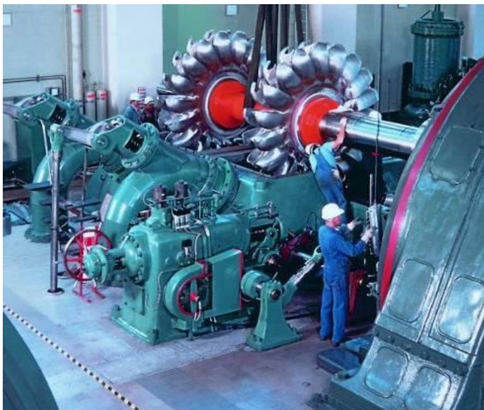
Figure E-5 A large utility-scale Pelton turbine installation (RenewablesFirst, 2015)
