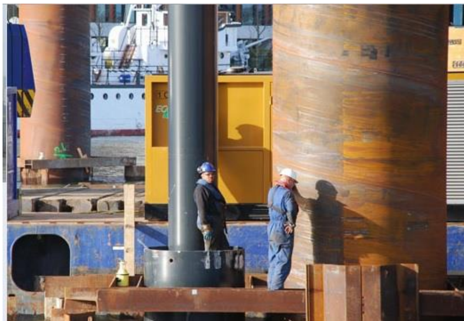
Figure D-6 Securing a steel pile with a diameter of 2400 [mm] in the port of Rotterdam (Gebr.deKoning, 2016)
