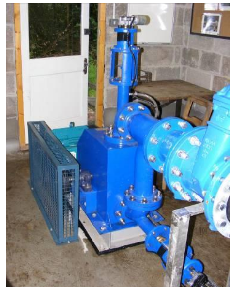
Figure E-6 A 11 [kW] Pelton turbine installation (RenewablesFirst, 2015)
