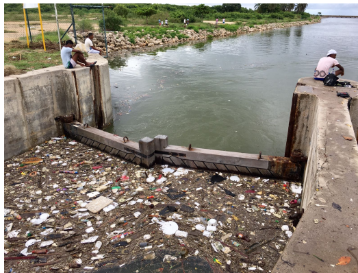
Figure 2.32: Garbage at the La Bocana water gate
