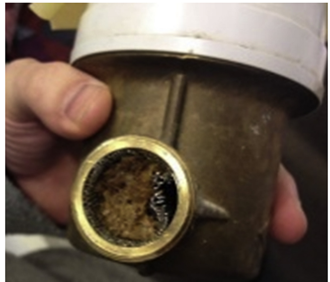
Fig. 4. Picture of particulate matter that clogged the water meter in Oasen's Hendrik Ido Ambacht supply area.
