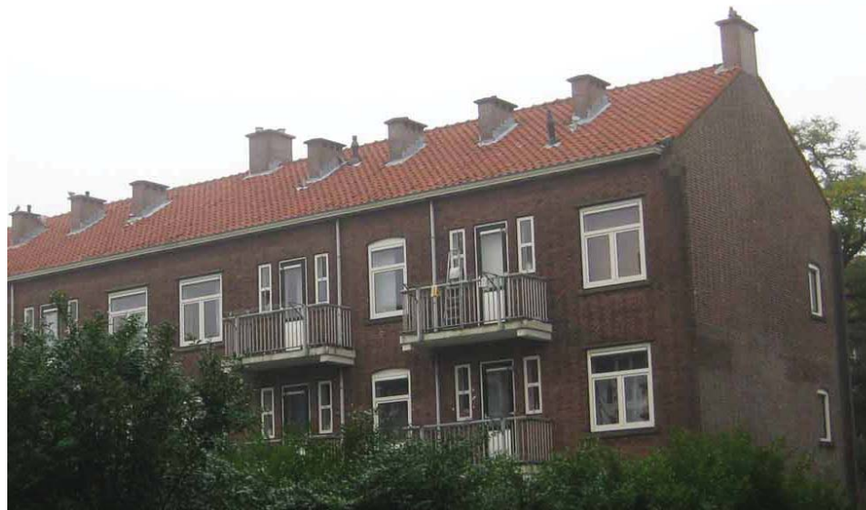
Fig. 78 : Photo by the author. Rear facade of VvE with 36 households in the Fazantstraat
