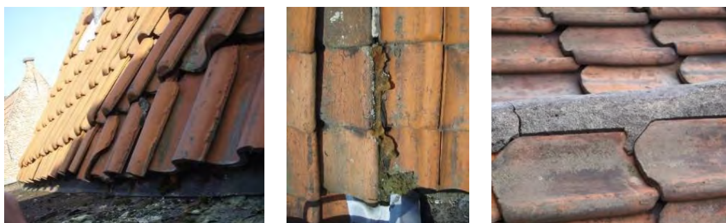
Figure 3: Left : lack of tile lath, resulting in shifted tiles, Centre : repair of connection with building foam, Right : hard mortar at connection between tiles, resulting in cracks and loss of connection. Pictures of case study by Monumentenwacht
