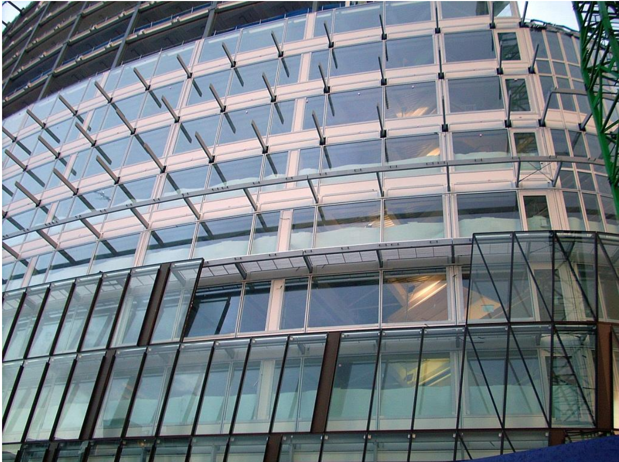
Figure 2.1: One Angel Square, Manchester, England. Detail of the double skin façade (during construction) that increases natural ventilation. There is a walkway between the inner and exterior façade panels for maintenance and solar shading.
