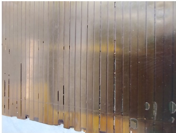
Figure 4.6: Close up to the voids in-between the pultrusions
