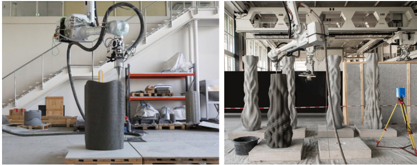
Figure 2.2: (a) Diagram of set-on-demand printing system, adapted from [16]; (b) Photographs of the set-on-demand printing system and printed columns at ETH Zürich, adapted from [17].
