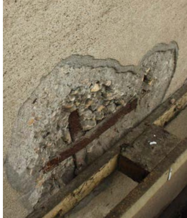
2 Corrosion of the reinforcement
