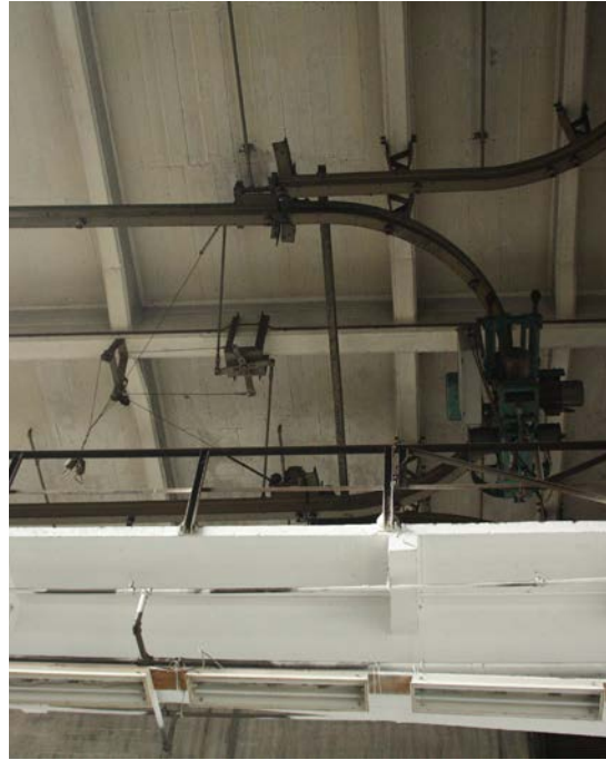
Image 2 - Rail changing system and operating cables
