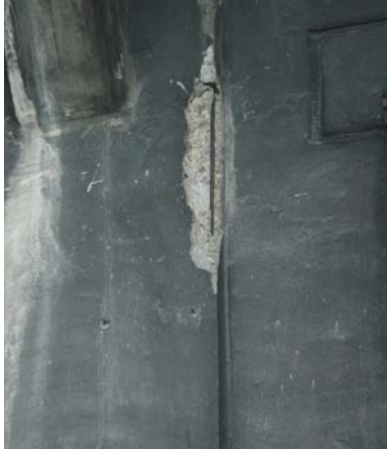
1 Spalling of concrete
