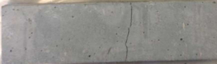
App. E - Figure 2 Crack Pattern of specimens B.
