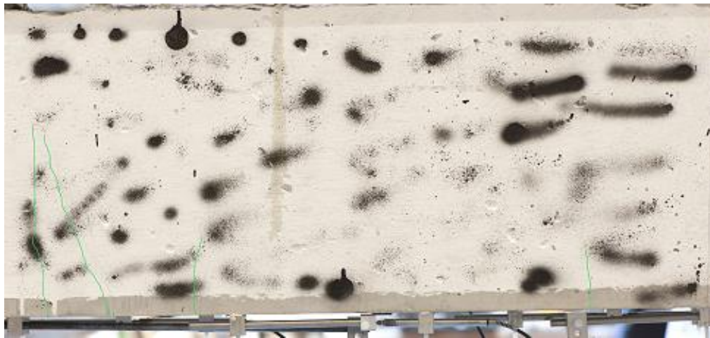
Figure 5.27 The displacement versus the pixel location (upper) for specimen FM2100-001, and corresponding picture of analyzed area with cracks highlighted with green lines (lower).
