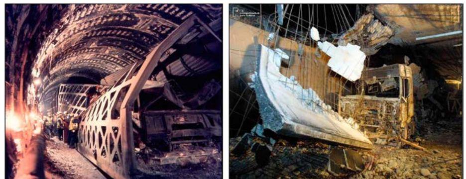
Fig. 1: (a) Damage to the concrete lining of the Channel Tunnel after the fire on 18 November 1996 (picture by Eurotunnel); (b) partial collapse of the ceiling of the Gotthard Tunnel after the fire on 24 October 2001 (picture by Ti Press)
