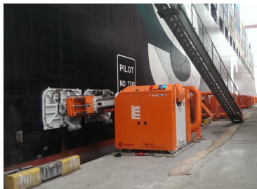
Figure 2.28: MoorMaster units in Port of Salah, Oman (Cavotec, 2020)
