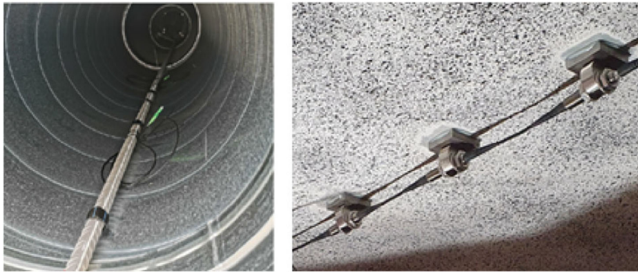
Figure 19. Application of FBG sensors. Left: glued to steel rebar, and right: attached to a concrete surface.
