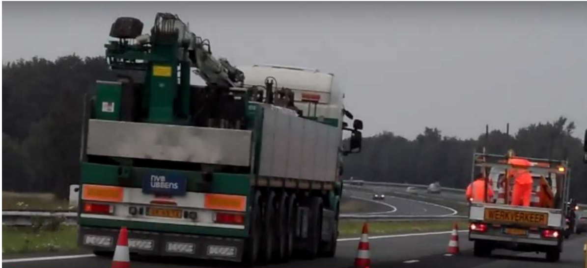
Figure 4.4: Example of placing traffic management measures on a Dutch motorway (source: handels- en Verhuurbedrijf Krans B.V.)
