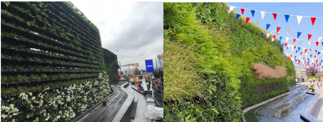
Figure 66: Installation of the green façade and opening day Gsky (N.D.) Westfield mall retrieved at 18-05-2020 from: https://gsky.com/portfolio/westfield-mall-london/
