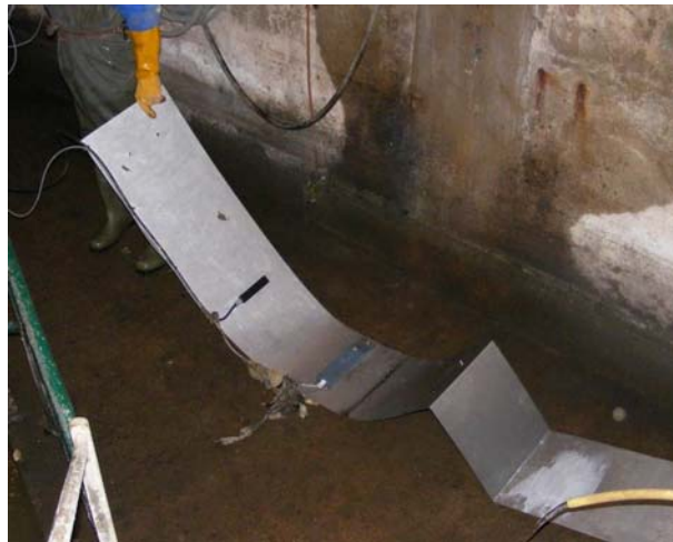
Figure 3.24 An ordinary Doppler sensor (left side, black sensor) and a Doppler profiler (right side, blue-grey sensor) during a comparison campaign. Note the tissues clogging on the connecting wires. Source: Université Gustave Eiffel.
