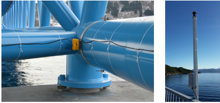
Figure 3: Left: accelerometer mounted on the truss; right: GNSS rover station at the middle of the bridge.
