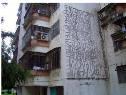
Deterioration (Source: bbs.szhome.com)
