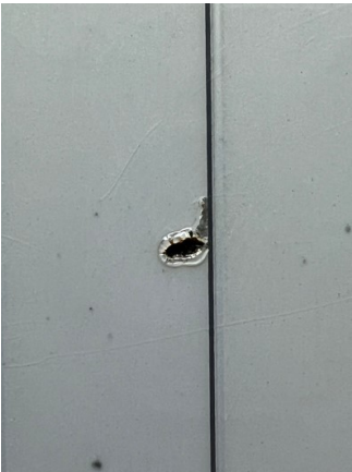
(b) Backside image of a hotspot created during WCSS on R20026-4096
