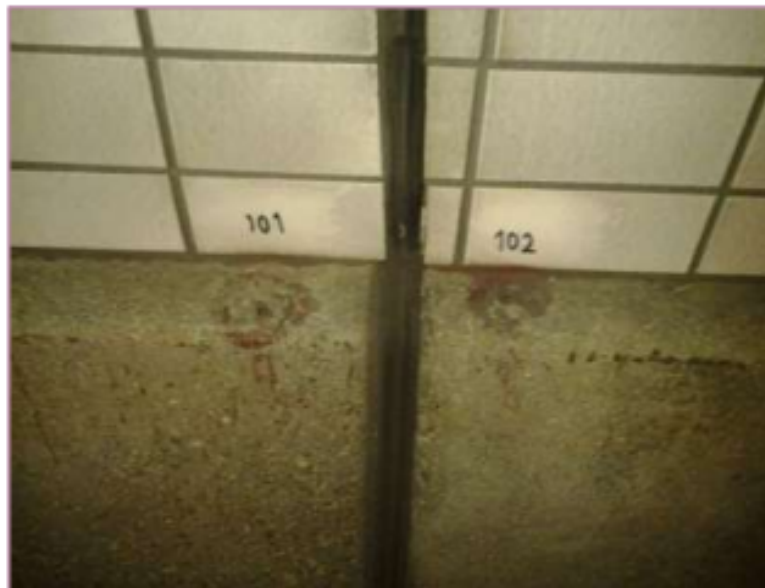
Figure 6.12: The measuring bolts (number 101 and 102) for regular measurement at immersion joint 1 (SWECO, 2020)
