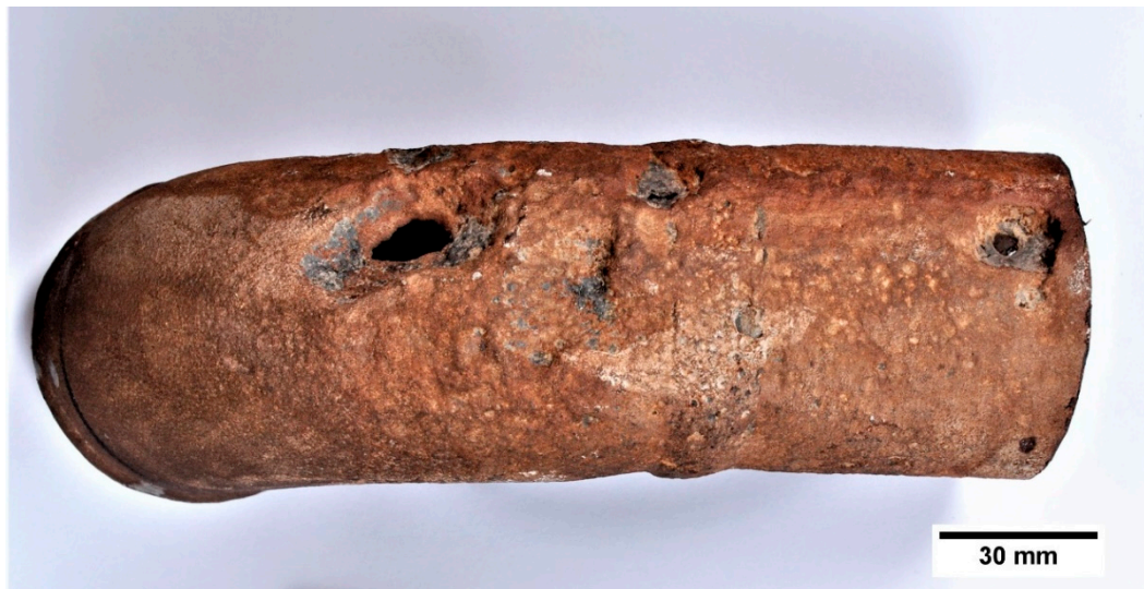
Figure 2. An example of the failed elbows.
