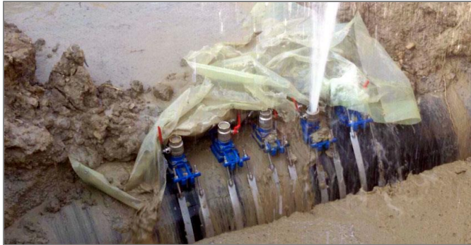
Figure c. Example of illegal connections to public water network in the area of Gela. The illegal withdrawal rate amounted to 30 l/s per connection. Source, regional newspaper http://www.quotidianodigela.it/images/luglio2016/allacci.jpg
