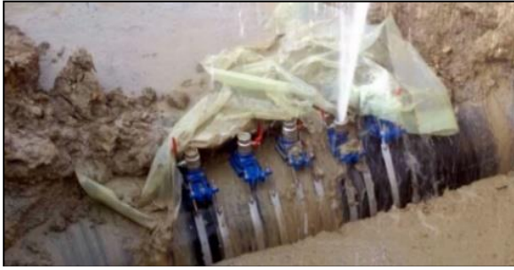
Figure 3: Example of five illegal connections to a public water network in Gela. The withdrawal rate amounted to 30 l/s per connection ††
