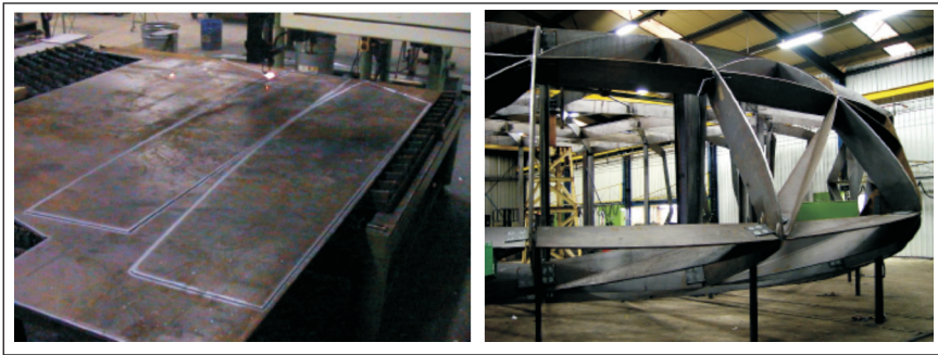
Figure 4.5: The production of the steel frames a) Left: The CNC-cut frames b) Right: Assembling the structure in the factory
