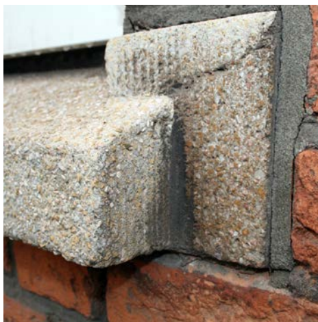
Figure 7.35 Prefabricated coloured concrete window sill; the texture has already partially eroded (housing, Rotterdam, exacts date and architect unknown, 1930s, situation 2010).
