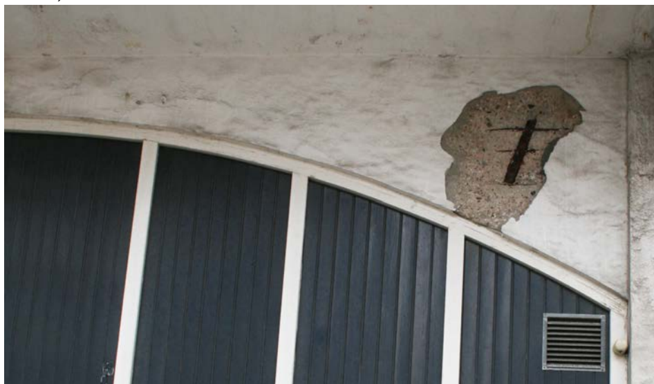
Figure 8.18 Example of an arch without the original surface. Instead a smooth, grey render was applied and painted white. The original reinforcement is visible due to local damage, notice the rectangular strips and horizontal plain round bars (Hofplein railway viaduct 1900-1908, situation 2012, compare also Figure 6.22).
