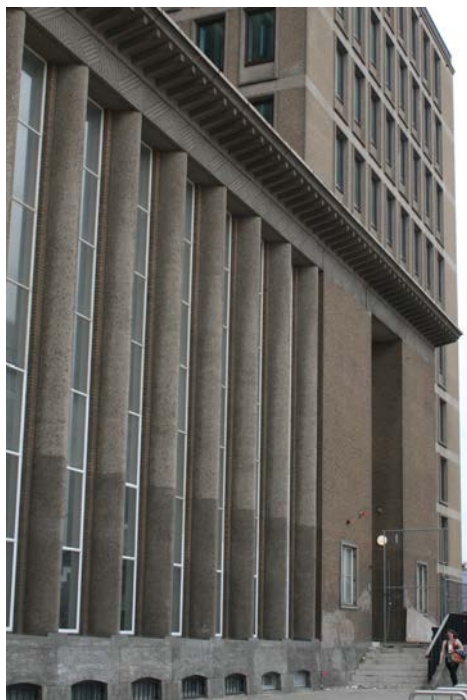
Figure 9.22 Example of the visual impact of anti-graffiti coatings: the lower zone of the façade was treated and is clearly distinguishable from the untreated upper zone (Former tax office, Amsterdam, G. Friedhoff and M. Bolten, 1954–1958, situation 2011).
