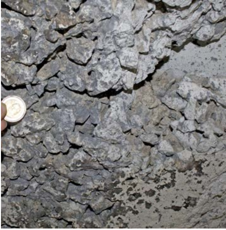
Figure 11.4 Example of honeycombs; plain concrete wall with crushed rock, cut through during a previous intervention (Fort near Hoofddorp, 1904, situation 2006).
