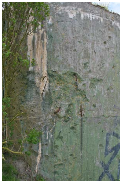
Figure 8.11 Damage caused by impact of shells during the Second World War (kanonkazemat VI, 1932, Defence line Kornwerderzand, situation 2009).
