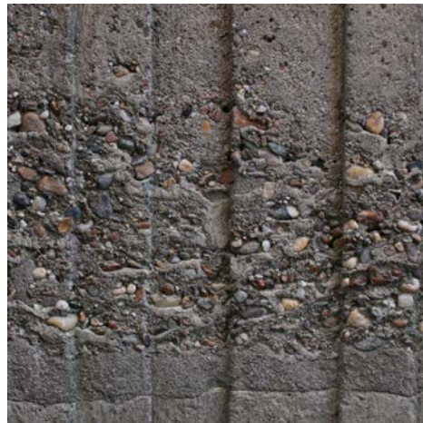
Figure 4.6 Example of use of gravel for exposed concrete; the gravels are locally visible due to segregation of the concrete during construction (Pumping station Parksluizen, Rotterdam, G. J. van der Grinten, 1967, situation 2008).
