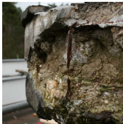
Figure 8.9 Loss of entire cross section of a reinforcement bar and parts of the concrete bulk (Dresselhuys pavilion, Hilversum, J. Duiker, B. Bijvoet and J. G. Wiebenga, 1928, situation 2008).
