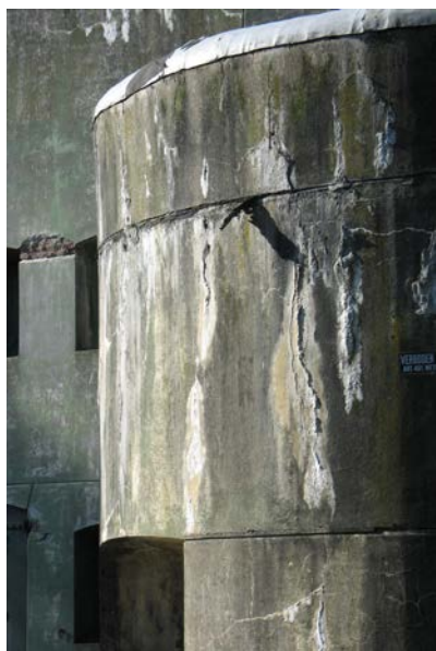
Figure 8.10 Deposits caused by leaching and cracking (Fort near Hoofddorp, 1904, situation 2006).
