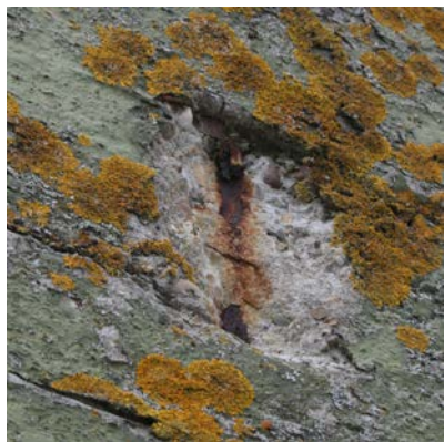
Figure 8.8 Biological growth on concrete surface, spalled concrete and corrosion (casement V, Defence line Kornwerderzand, 1933, situation 2009).
