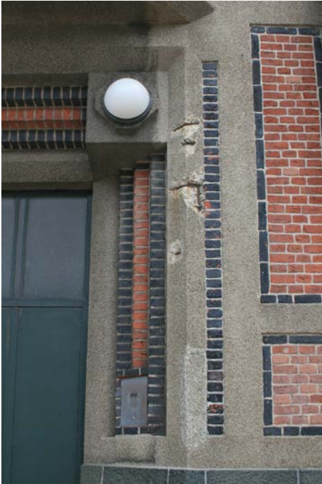
Figure 8.3 Example of a modified surface: the original surface was sand blasted, but has been covered with a render with pebbles, and with local later repairs and spalling (office building De Nederlanden van 1845 , The Hague, H.P. Berlage; 1921 -27, situation 2009).
