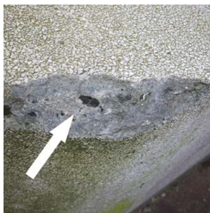
Figure 7.75 Decorative concrete element, due to damage of the facing layer and backing layer are visible; the facing layer was made with one type of small crushed stone; notice their greyer colour at the fractured surface (social housing, Rotterdam, M. J. Granpré Molière P. Verhagen, 1935, situation 2010).
