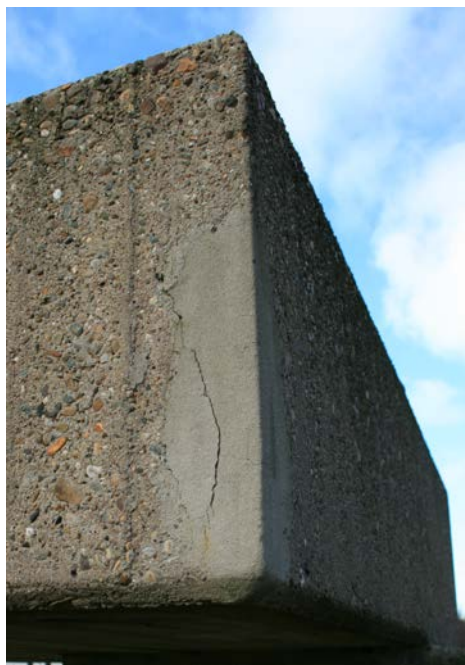
Figure 9.17 Corner of an exposed concrete sculpture showing a cracked repair mortar with rust stains, indicating ongoing corrosion (sculpture by C. Visser, TU Delft, 1966, situation 2006).
