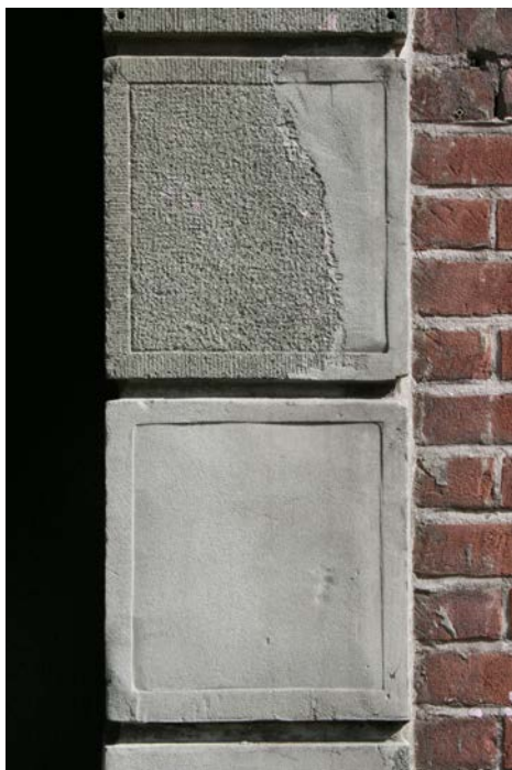
Figure 9.12 Concrete made with diabase as aggregate and bush hammered surface with chiselled margins which was repaired with a grey, smooth repair mortar (housing, 1930s, exact date and architect unknown, Rotterdam, situation 2011).
