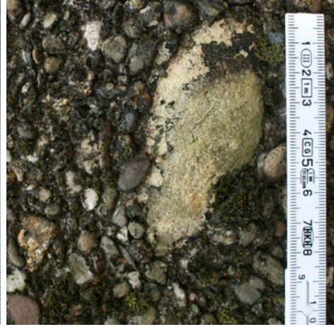
Figure 4.17 Local deviation of maximum aggregate size, the maximum size should have been 60 mm (earth retaining walls of the unfinished Groot Museum Kröller - Müller, national park Hoge Veluwe, H. van de Velde, 1921-1922, situation 2008).
