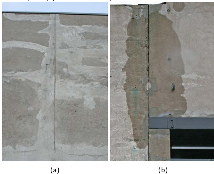
Figure 11.3 Two different interventions of the active cracks caused by thermal movement. a) Example of a failed repair of an active crack: the concrete was injected and new expansion joint created and filled with an elastic sealant; yet, the cracks reappeared (Fort Bezuiden Spaarndam, 1897-1901, situation 2006). b) Example of an untreated crack showing the risk of moisture ingress (dark zone is moisture, visible after a rain shower); the parapet has not been covered, allowing additional moisture ingress from the top (Fort near Vijfhuizen, 1899, situation 2008).
