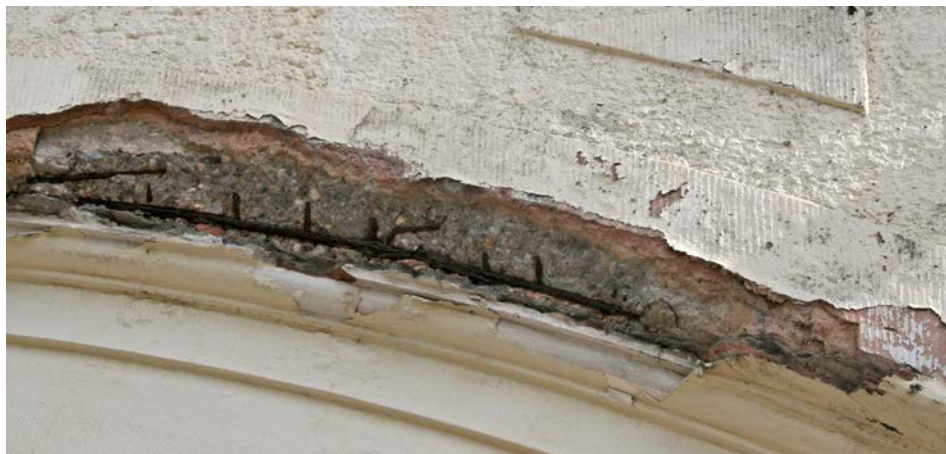
Figure 8.17 Example of local damage of render and concrete, exposing the reinforcement, in this case round bars and round stirrups (Hofplein railway viaduct, situation 2009).
