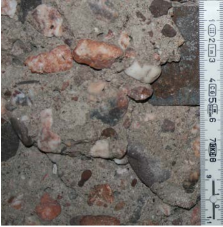
Figure 4.16 Gravel used for columns at the Hofplein railway viaduct; originally intended were 5 and 25 mm large aggregates, yet local deviations can be encountered. The pink discolouration of the aggregates was caused by a fire during the bombardment of Rotterdam in May, 1940. (Rotterdam, A. C. C. G. van Hemert, 1900-1908, situation 2009).
