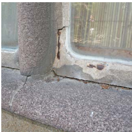
Figure 7.3 Prefabricated coloured concrete elements; due to local damage it can be seen that the material is concrete and not a render (Riveràhal of the Zoo Blijdorp, Rotterdam, van Ravesteyn, 1939-1941, situation 2011).
