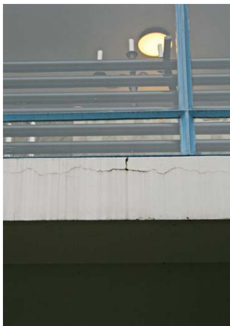
Figure 9.16 Detail of a corner of a concrete slab, the repair mortar has cracked in less than 6 years after repair and is visible due to soiling (Sanatorium Zonnestraal, Hilversum, J. Duiker, B. Bijvoet and J. G. Wiebenga, 1928, restoration began in 2001, situation 2007).
