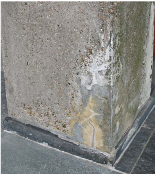
Figure 9.8 Column of an exposed concrete repaired with a polymer-based patch repair, showing discoloration due to ageing (Faculty of Architecture, TU Delft, architectural firm van de Broek & Bakema, 1960-1970, building burnt 13.05.2008, situation 2007).
