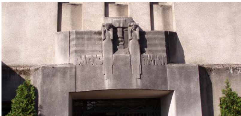
Figure 7.61 Entrance Radio Kootwijk, relief made in-situ by using gypsum formwork. The colour difference between the entrance and the walls behind is not original, but caused by the application of sprayed concrete in the 1960s on the walls (J. M. Luthmann, J. Emmen, artist H. van den Eijnde, 1921-22, situation 2006).
