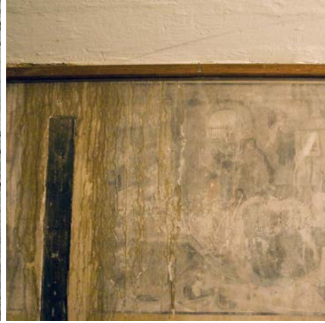
Figure 11.5 Example of seepage through former construction joints and cracks caused by thermal stresses in the interior of the fort (Fort Bezuiden Spaarndam, 1897-1901, situation 2006).
