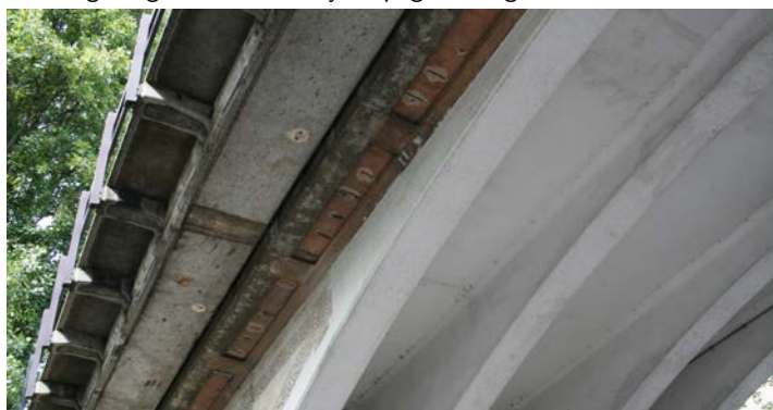
Figure 8.20 Example of different interventions and resulting surface finish: the soffit shows a grey concrete from 1950s extension, next to it an original reddish stripe of render with locally exposed reinforcement and the white painted intrados with local repairs without texture (Hofplein railway viaduct 1900-1908, situation 2012).
