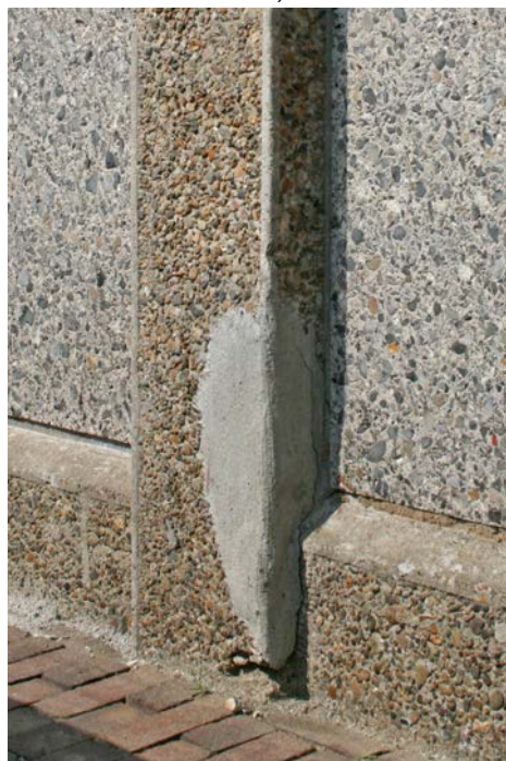
Figure 9.13 Column with exposed aggregate surface finish and standard grey patch repair (Train station Zutphen, H.G.J. Schelling, 1952, situation 2009).
