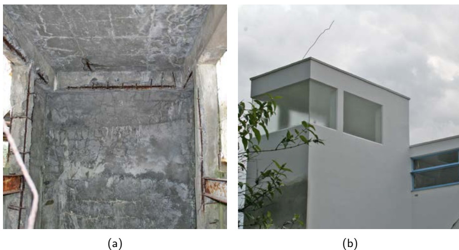
Figure 5.6 Example of corrosion induced by chlorides which were cast in to allow works during low temperatures. The historic concrete structure was demolished and reconstructed ( Dresselhuys pavilion , part of Sanatorium Zonnestraal , Hilversum, J. Duiker, B. Bijvoet and J. G. Wiebenga, 1928). a) Interior view of lift shaft before demolition, showing exposed reinforcement, cracking and efflorescence (January 2008). b) Exterior view of the reconstructed lift shaft (September 2008).
