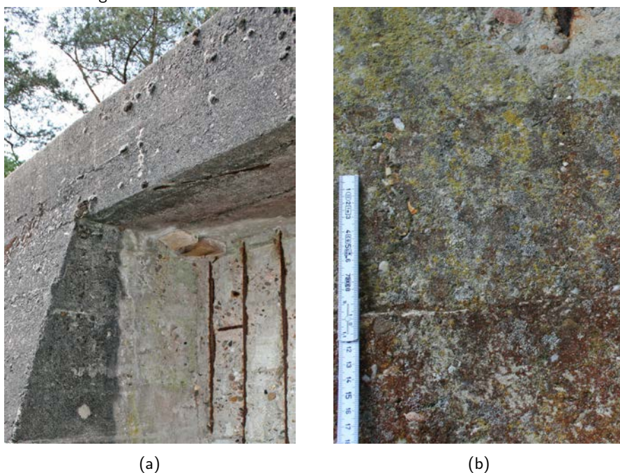
Figure 8.29 Signs of merging with the landscape and local degradation (Groot Museum, Natural park Hoge Veluwe. H. van de Velde, 1922, situation 2008). a) Colour variation of the concrete caused by biological growth, and local spalling of the concrete; notice the remains of the original formwork in the corner. b) Colour variation of the concrete caused by biological growth.
