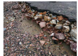
Collapsed road due to heavy trucks
