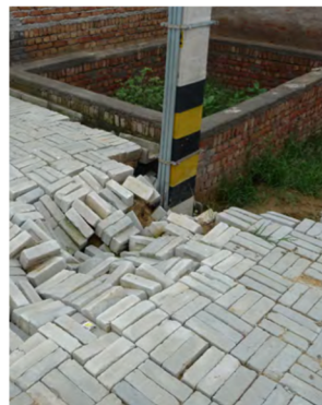
Poorly made street surfaces collapse
