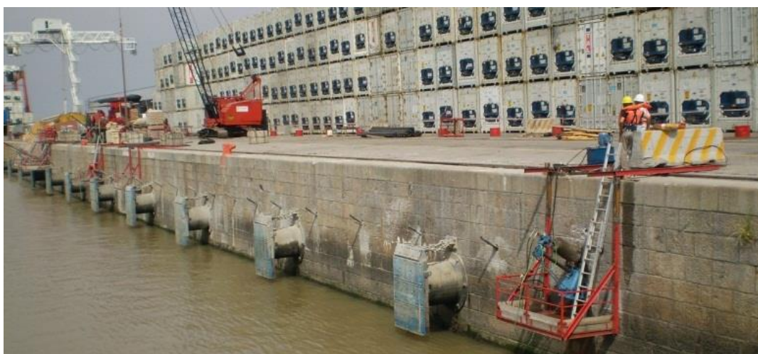
Figure 4-2 Active post-tensioned anchors to reinforce existing quay walls at Port of Buenos Aires
