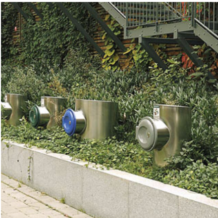
view of vacuum waste system stations
