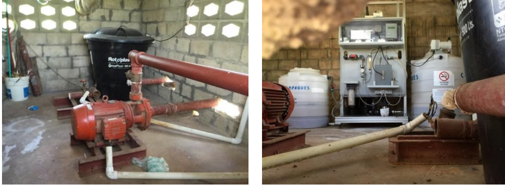
Figure 24: Water pump (right) and disinfection method (left).
