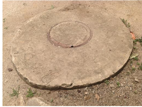
Figure 30: Inspection chamber of the sewage system in Palomino.
