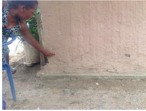
Figure 32: Women showing the flood level on rainy seasons in the neighborhood 'El Divino Niño'. Approximate 15 cm was measured.
