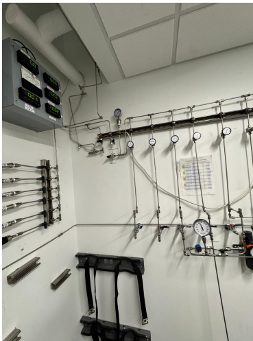
(d) Additional pressure transducers and gauges
