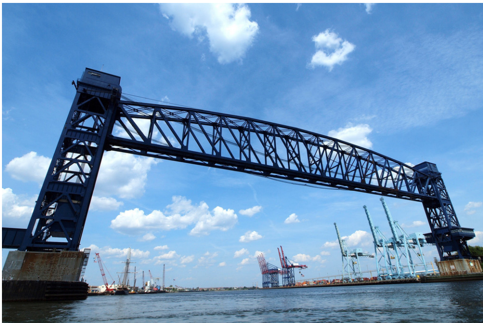
Figure 5.31: The Arthur Kill Vertical Lift Bridge is a railroad only vertical lift bridge which connects Staten Island and New Jersey via a 170 meter long truss span (Wikimedia Commons, 2006)
