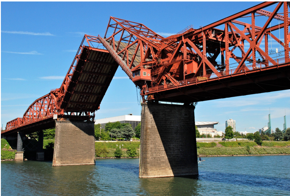
Figure 5.26: The Broadway Bridge in Portland, OR crosses the Willamette river and features a double-leaf bascule bridge (Wikimedia Commons, 2009)
