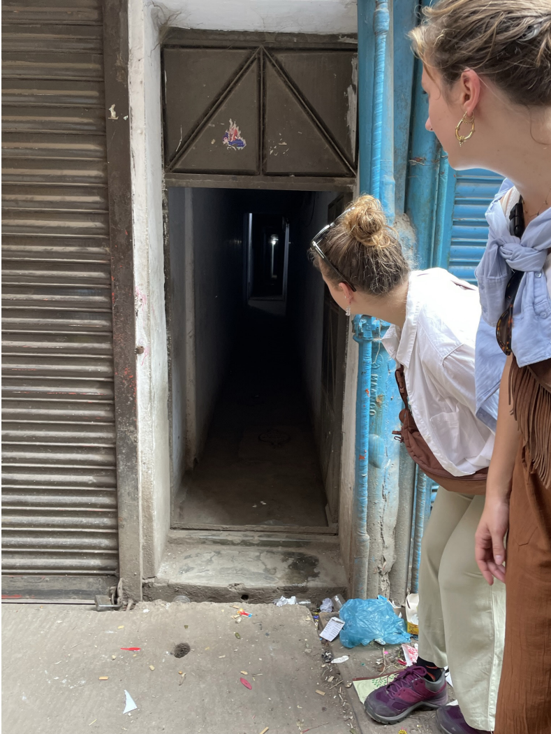
Inadequate living space with minimum daylight entrance and no fire safety Source: Own photograph
