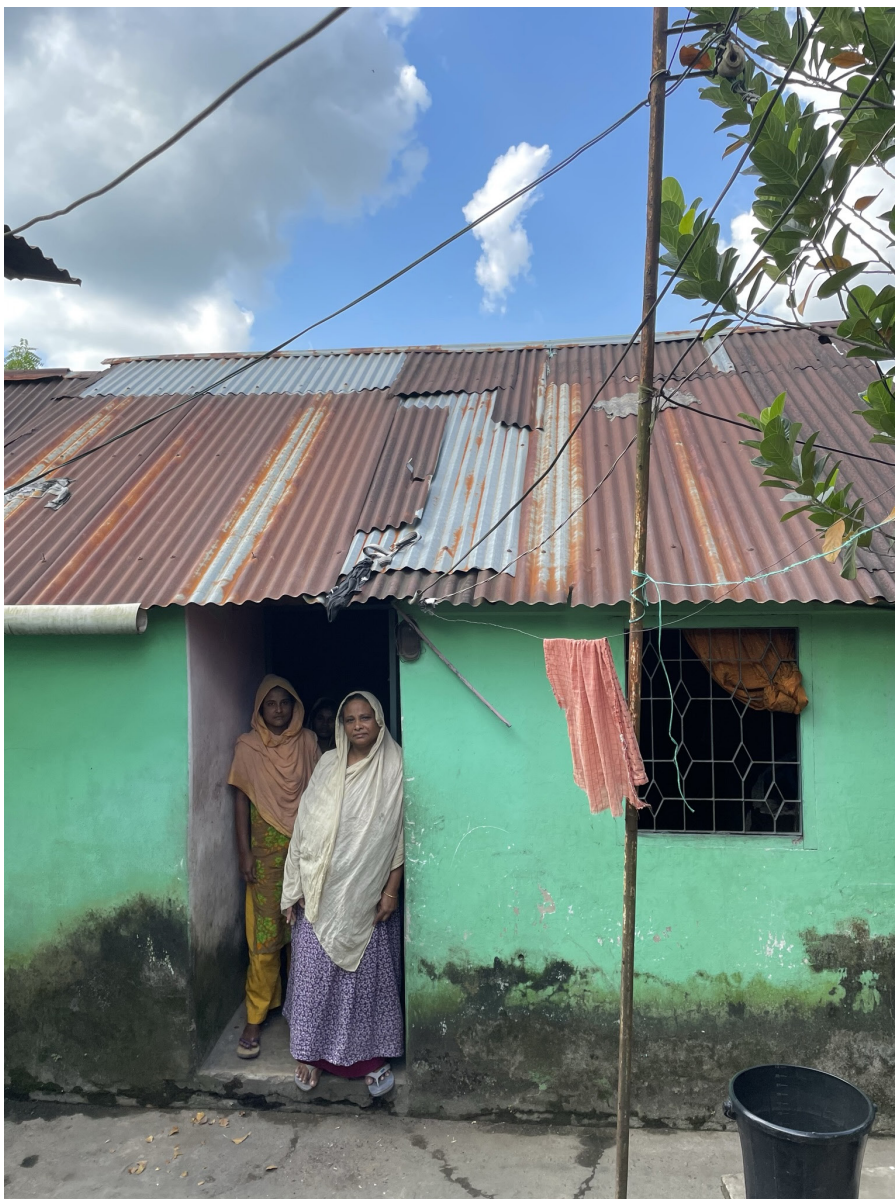
Housing in informal settlement in Laladighir Par, Sylhet Showing the water level marks during floodings in the monsoon season Source: Own photograph
