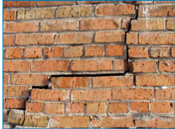
Figure 18: Lowering the groundwater table can result in foundation settlements, resulting in damage ( http://www.profoundprofessionals.com )
