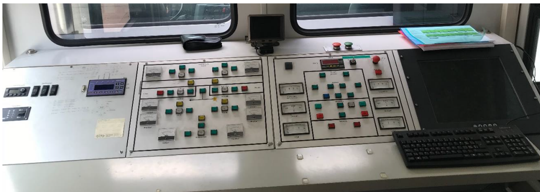
Figure 3.3: Console inside the cabin of MoreLab
