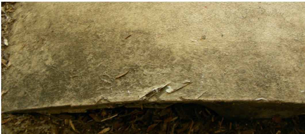
Figure 8. Edge of the blade already brittle, with glass fibres and parts of the coating exposed to the users (Photo by Piero Medici, 2011).
