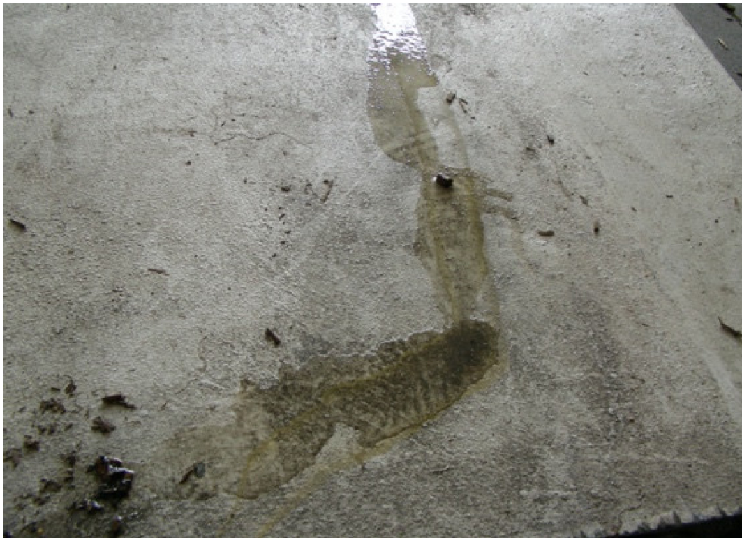
Figure 20. Blade lying horizontally working as a rain gutter, a yellow leach is visible (Photo by Piero Medici, 2011).
