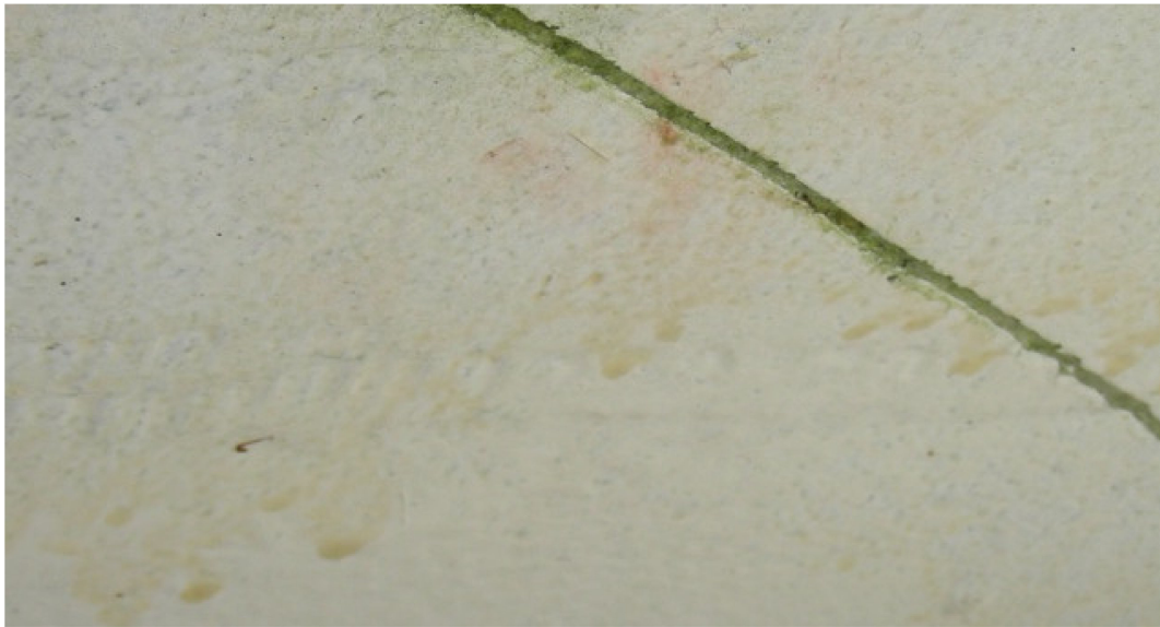
Figure 24. Close-up of the drops next to a surface opening (Photo by Piero Medici, 2011).
