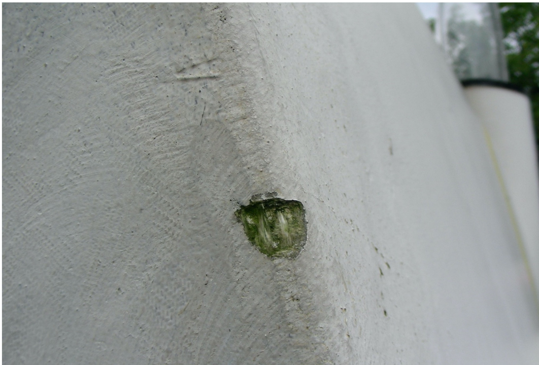
Figure 9. Damaged finish by Maropol, with glass fibres exposed, as a consequence of use damage (Photo by Piero Medici, 2011).
