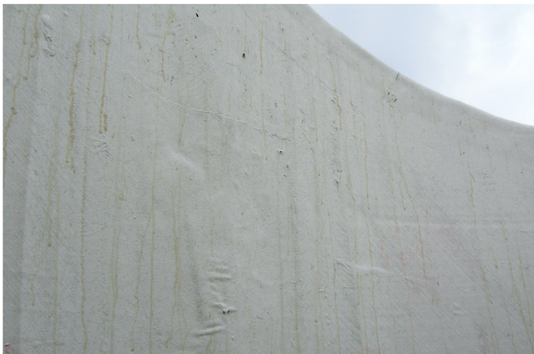
Figure 17. Leaching from the top of a tower (Photo by Piero Medici, 2011).
