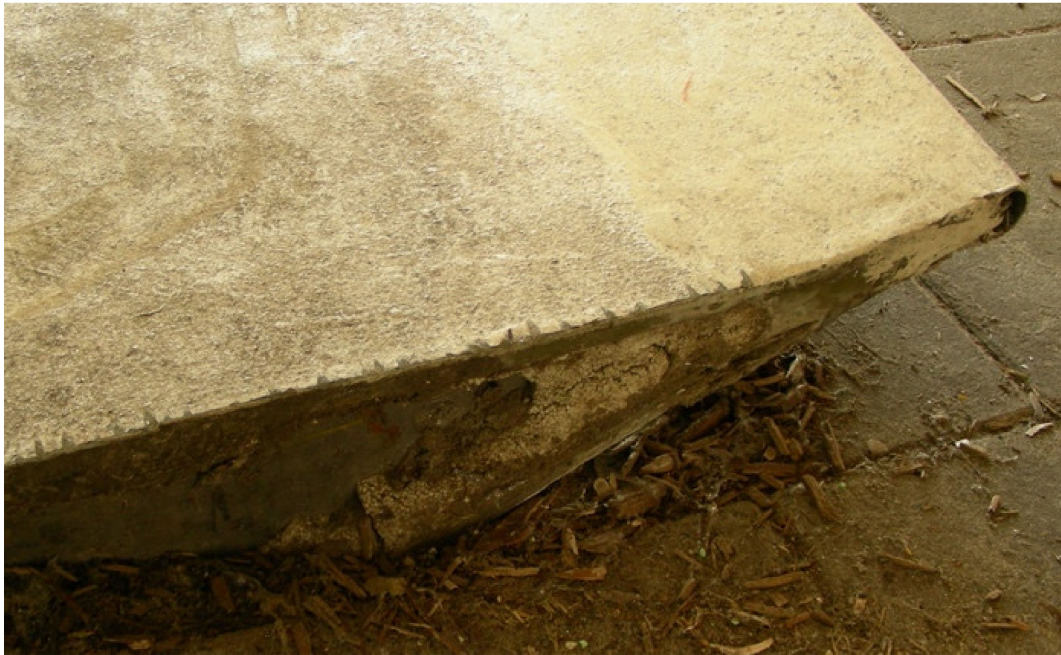
Figure 7. Edge of the rotor blade already brittle with polystyrene coming out, as a consequence of the users walking on it (Photo by Piero Medici, 2011).
