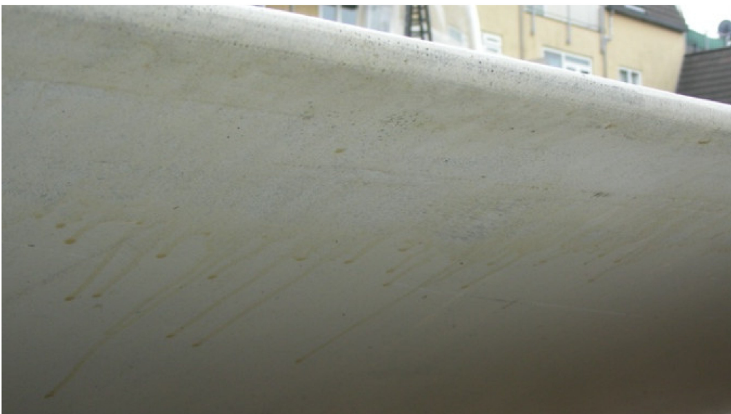
Figure 23. Leaching below a blade lying horizontally (Photo by Piero Medici, 2011).
