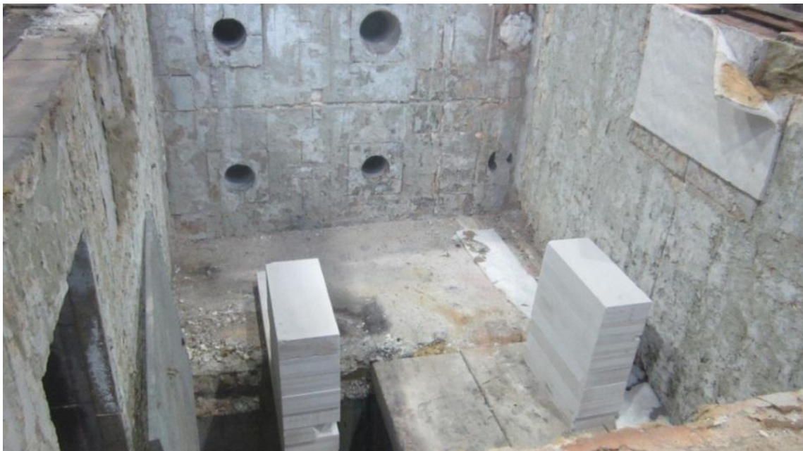
Figure 5.68 location of ACC inside the furnace
