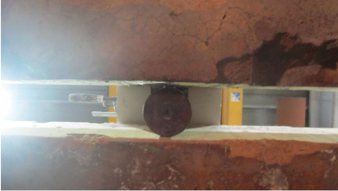
Figure 5.71 View over camera form inside the furnace
