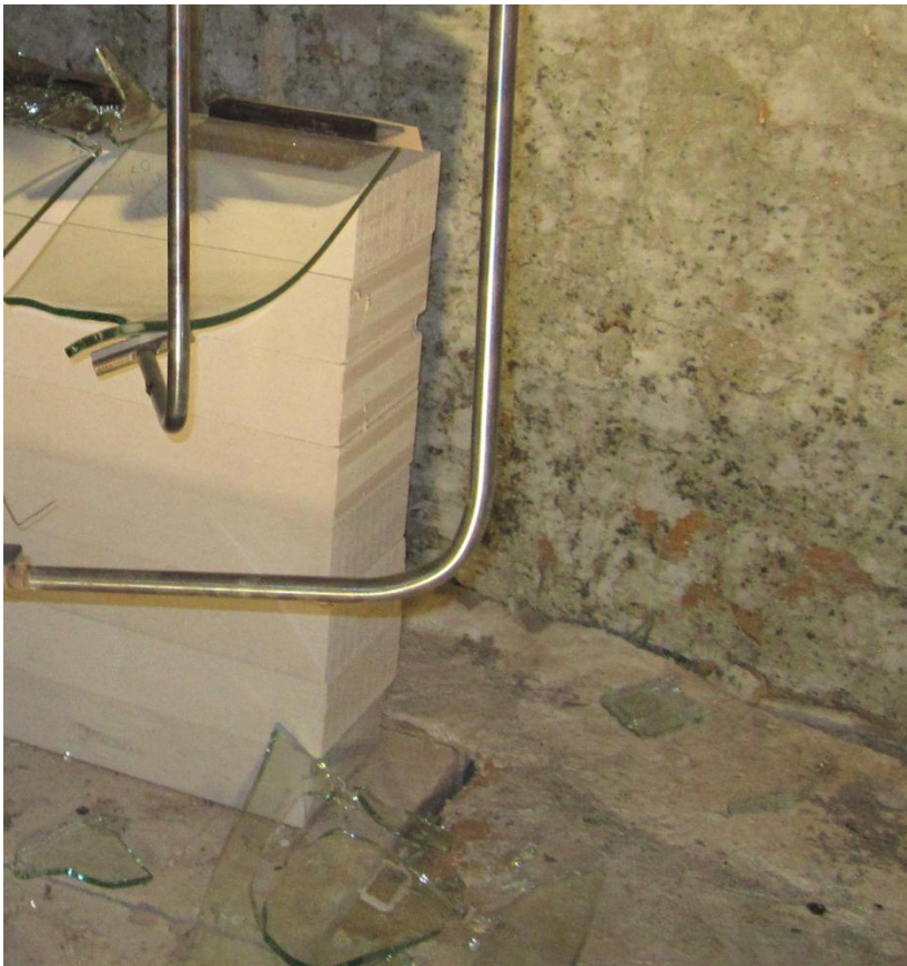
Figure 5.95 Pane fell down after thermal break
