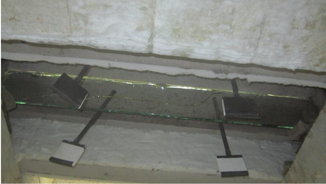
Figure 5.59 Pane D after break
