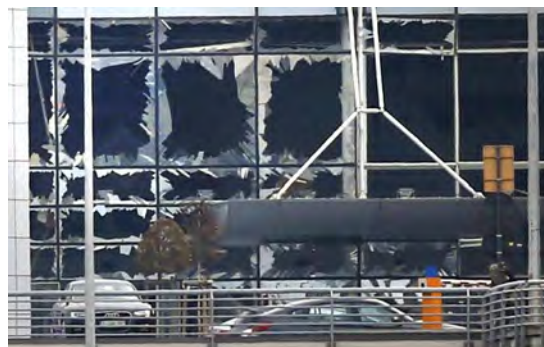
Facade of Brussels airport after the terror attack on 22.03.2016 [nzz.ch].
