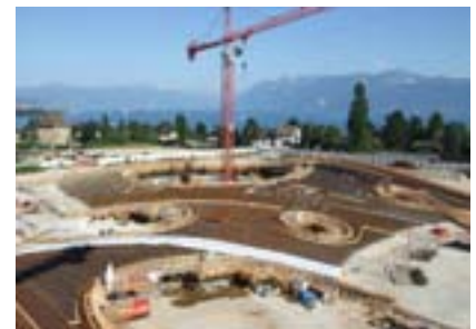
construction of the slab for the larger hill 2008 all pictures on this page from lecture of Grohmann 2008
