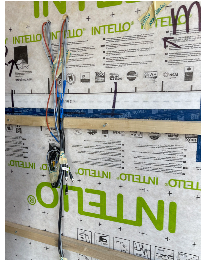
Figure 38: Monitoring equipment integrated in frames
