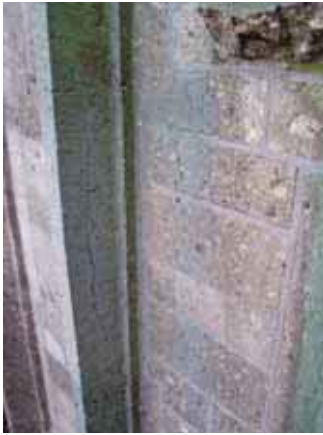
Figure 1. Ettringen tuff mullions showing damage in the form of longitudinal cracks (tower of Eusebius church, Arnhem, the Netherlands)
