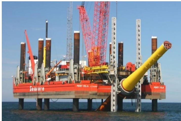
Figure 2.10: A barge from Fugro Seacore performing craneless monopile upending using a vertically translating frame and gripper [24].
