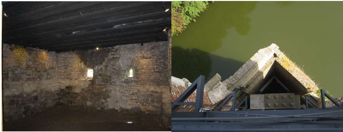
Figure 64- Overview at the left side of the prefab concrete floor at the cellar which substitutes the vaults and floors from the original construction. This consolidation was made at the 1 st consolidation works of 1975. At the right side it's the overview of the concrete ballast where the steel staircase is standing on (own pictures)
