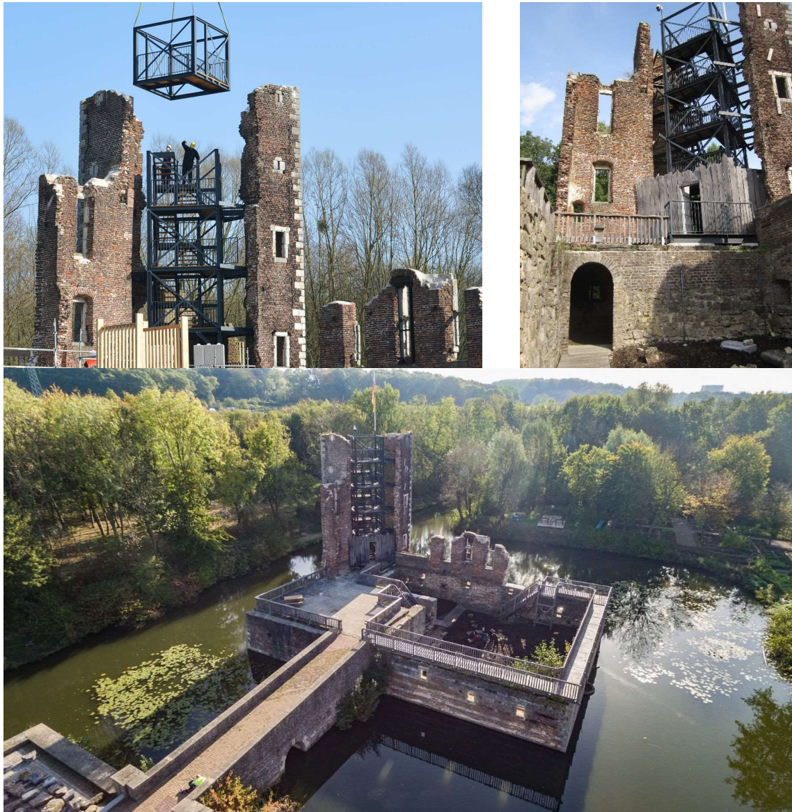
Figure 63- Overview of the construction of the steel staircase (on top left) and the ready done stage (at the other pictures)(Viersen, 2014)
