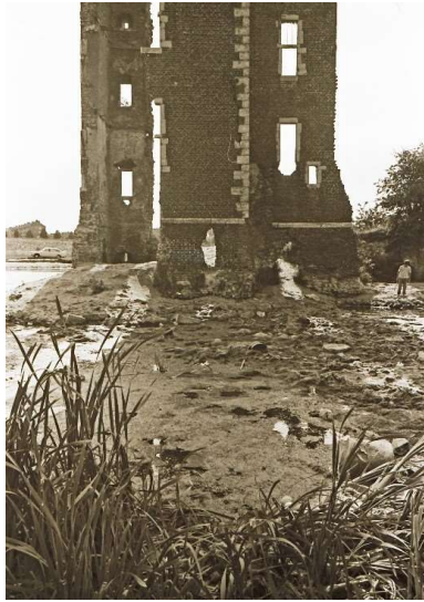
Figure 52- The lower part of the tower, viewed from the east, shortly after the southeast corner collapsed. The adjacent part of the east facade is also visible here (Photo: Hukkelhoven, Heemkundevereniging, (Viersen, 2014)
